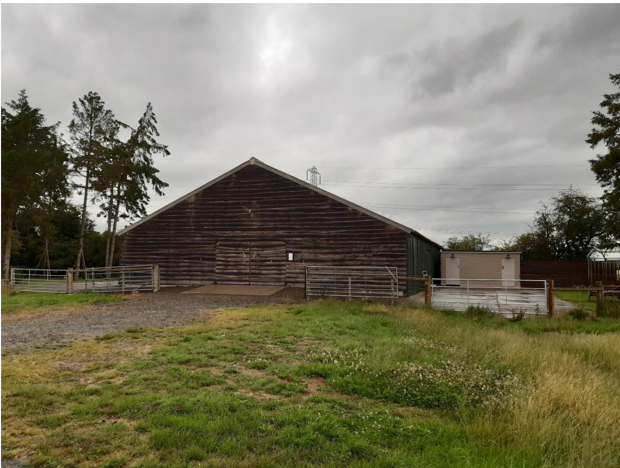
Figure 4 Front of the barn view from the outside, with large double door in the middle and toilets to the right.
